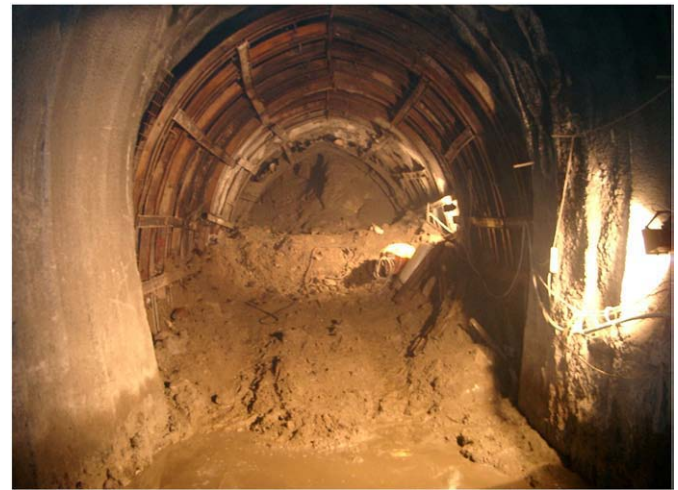
Fig. 10. Huge collapse as a result of remarkable amount of convergence in squeezing ground condition in Malatya Railroad Tunnel.
