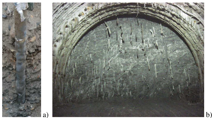
Figure 4. (a) P.E.R.Ground® bar removed after injection and (b) tunnel face improved by means of P.E.R.Ground®.
